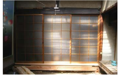
22.02.2005: The doors shut properly
