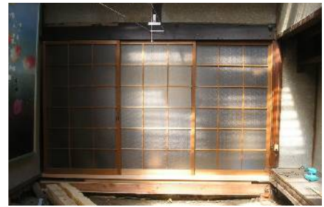
22.02.2005: The doors shut properly
